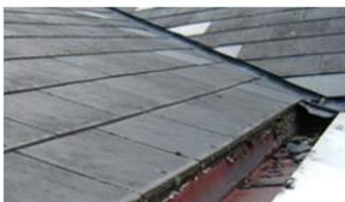
Roof tiles containing asbestos
