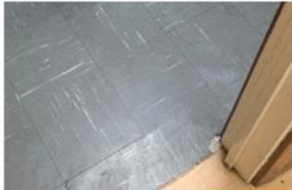
Asbestos in old floor tiling
