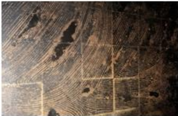
Asbestos in bitumen adhesives
