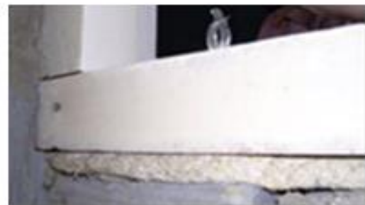
Asbestos rope packing under doorframe
