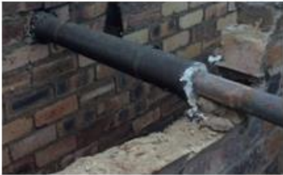
Damaged asbestos pipe lagging
